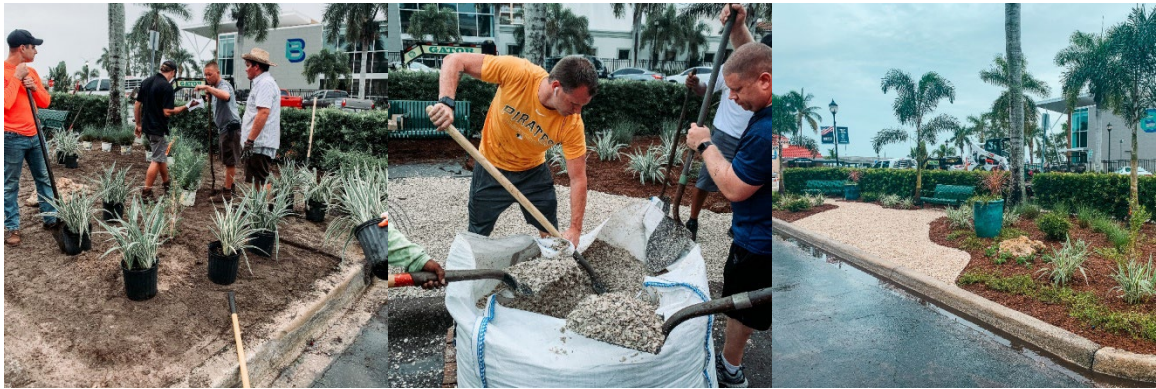
Many hands make for light work! Installing the new BPD outdoor lobby
